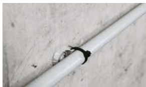
Flexible or rigid cable conduits with cable ties
