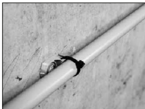
Flexible or rigid cable conduits with cable ties
