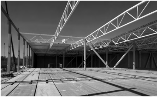
Figure 126. Steel hall construction with trusses made of steel grades up to S700M
